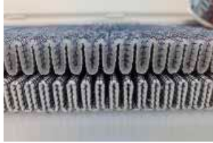
The filter media has absorbed water
